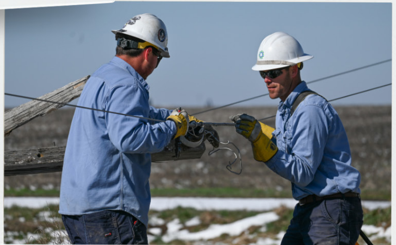
Line Repairs After Blizzard in Great Bend, Kan.
